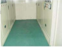
Low voltage room
