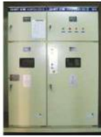
High voltage room
