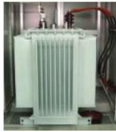
Low voltage room
